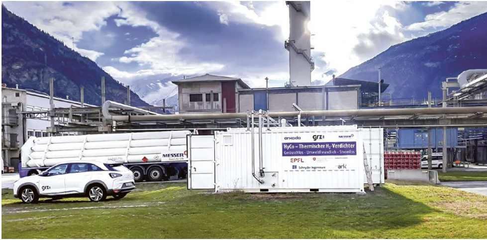
HyCo compressor installed at operational site
