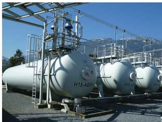
Hydrogen storage tanks (30 bar) at Djeva in Monthey.
