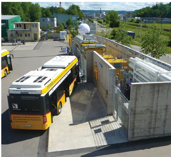
Hydrogen refilling station in Brugg (2011).
