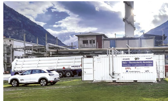
Metal hydrides hydrogen compressor HyCo with a capacity of 30 kgH 2 /h up to 200 bar developed by GRZ Technologies SA and installed in 2022 on the premises of Messer Schweiz AG on the site of Lonza/Arxada in Visp (Switzerland).
