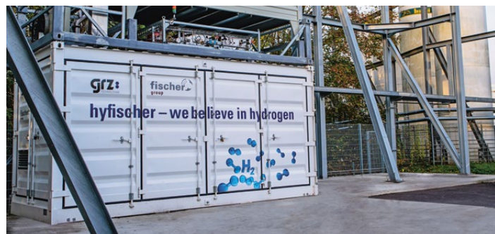
Figure 2 | DASH Power system commissioned at the Fischer Group, Achern, Germany.
