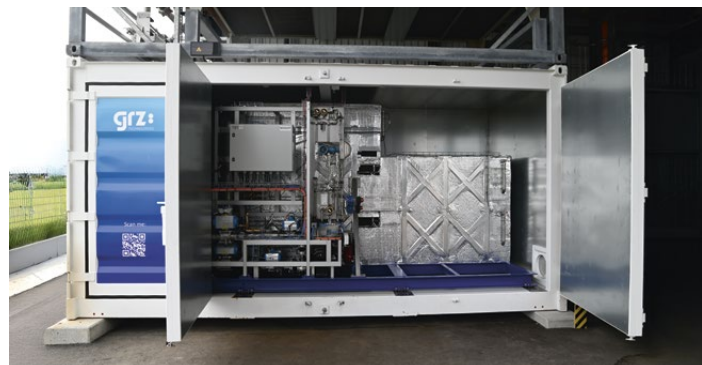
Figure 1 | DASH C-Series system commissioned at Gruyère Hydrogen Power SA, Bulle, Switzerland.
