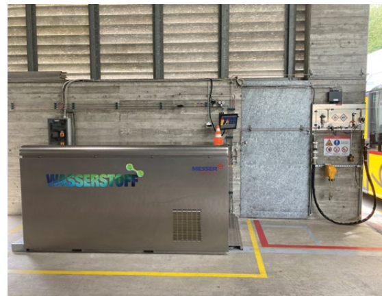
Hydrogen metal hydride based fuel station for forklifts at Messer in Lenzburg.
